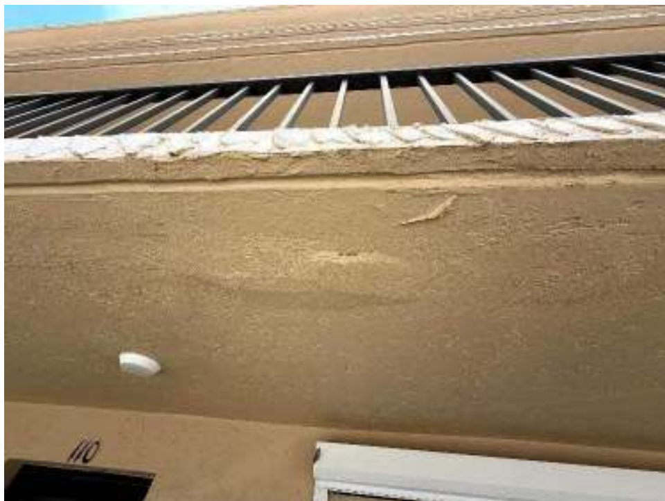
View of edge/ceiling spall along ground floor ceiling walkway
