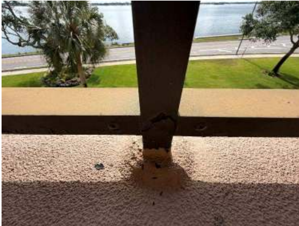
View of corroded cored railing with deteriorating coatings
