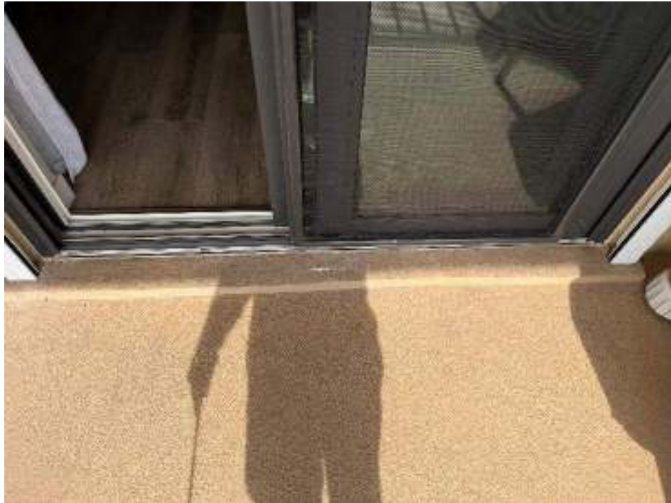
View of damaged floor coatings at sliding glass door threshold
