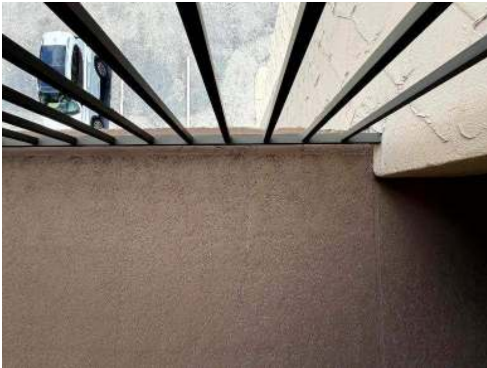
View of crack along walkway slab
