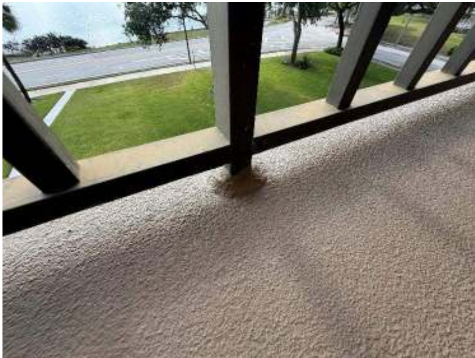
View of deteriorating railing coatings
