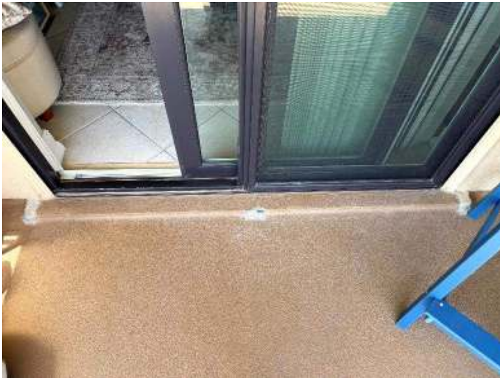
View of typical balcony coatings Note missing coatings where shutter frame was installed
