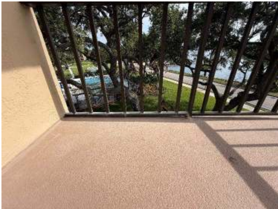
View of typical cored railing with deteriorating coatings
