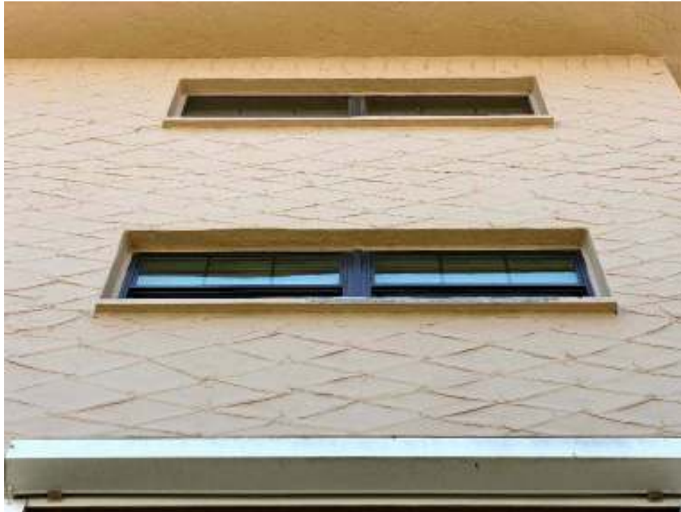
View of “patched” windowsill spall
