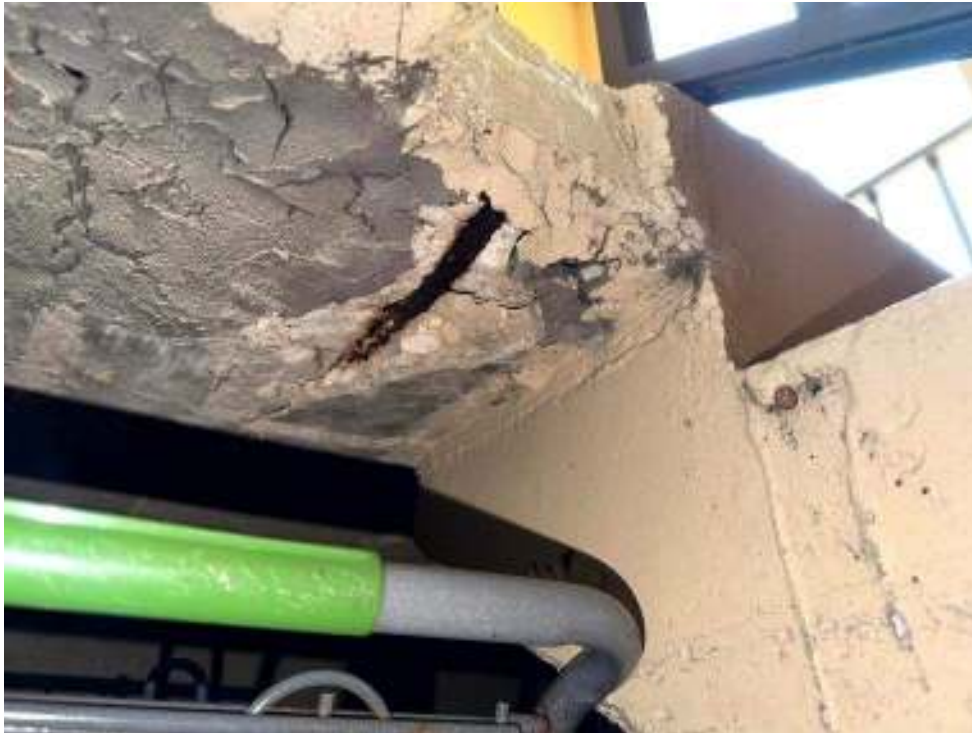
View of spall underneath stairs
