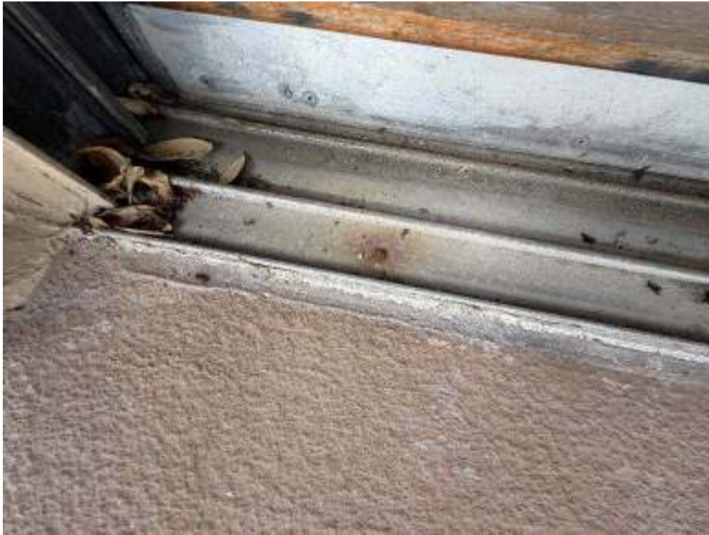
View of corroded sliding glass door fasteners
