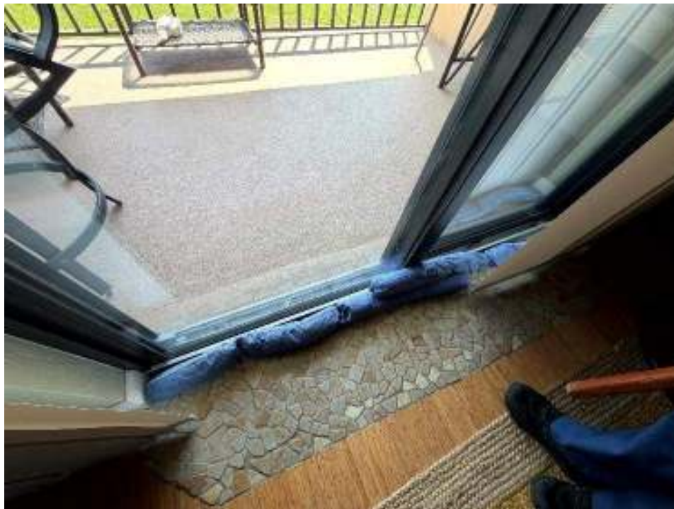
View of sliding glass door with possible water intrusion
