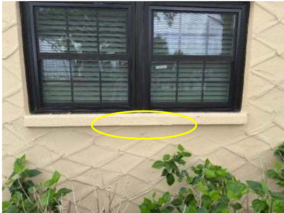
View of patched windowsill spall
