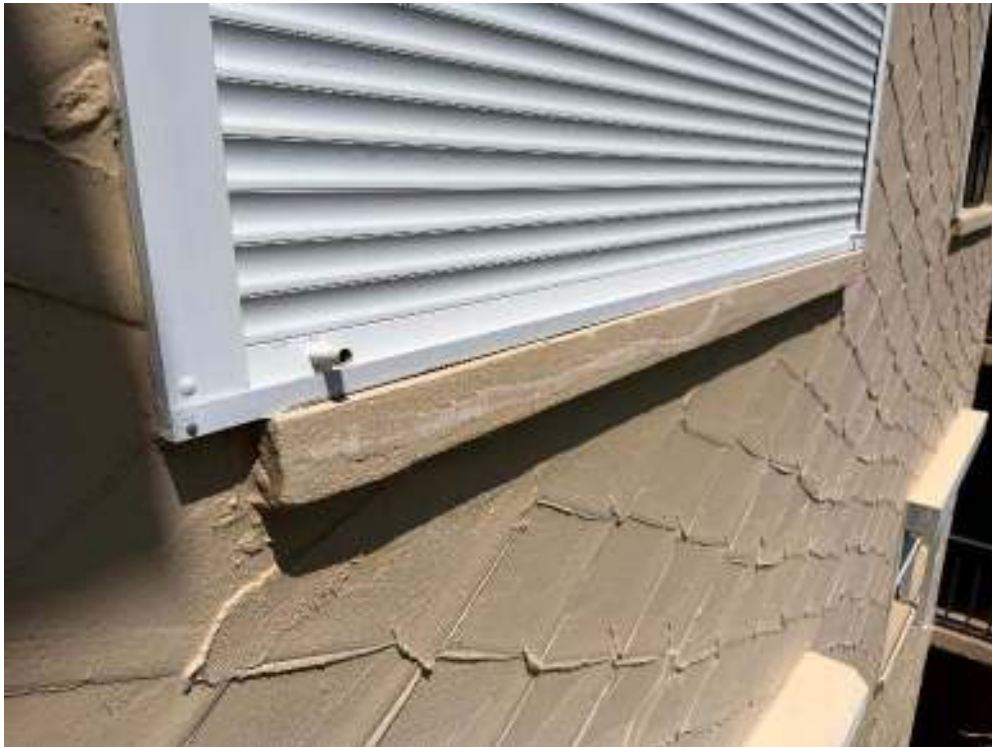
View of “patched” windowsill spall
