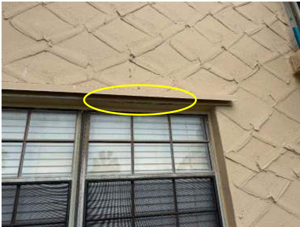
View of header spall above window
