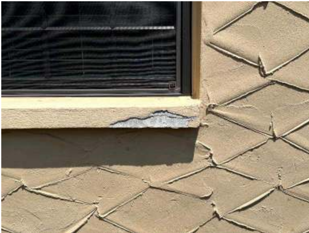
View of windowsill spall
