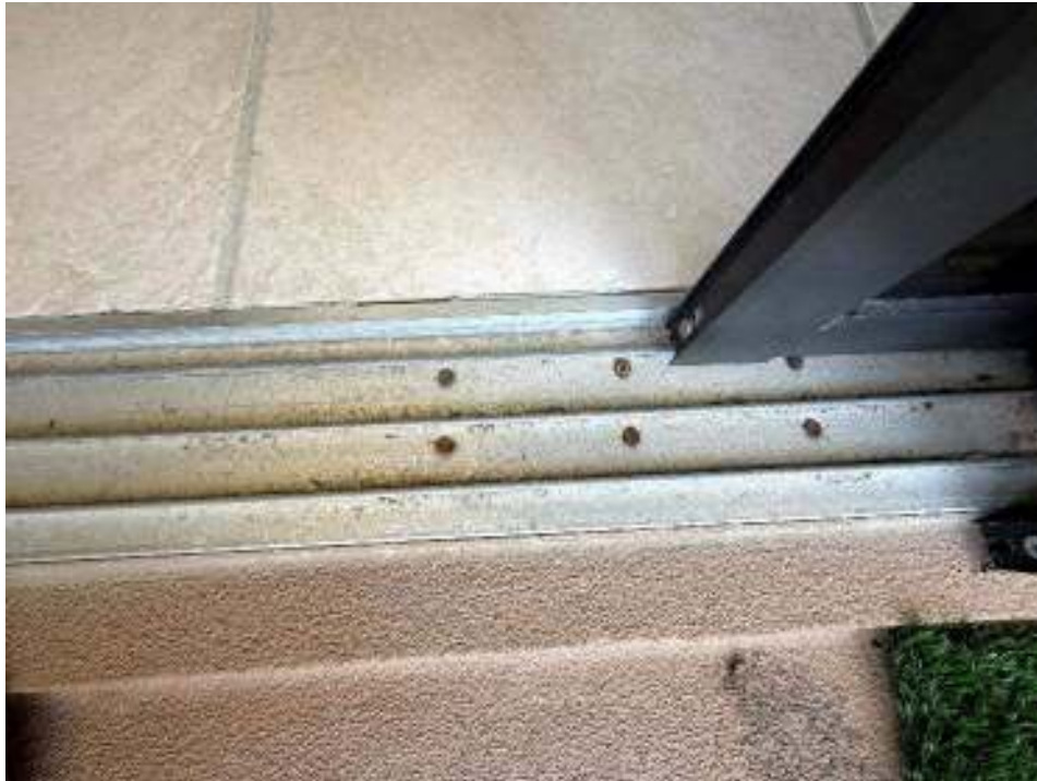
View of older sliding glass door Note corroded fasteners and deteriorating door coatings
