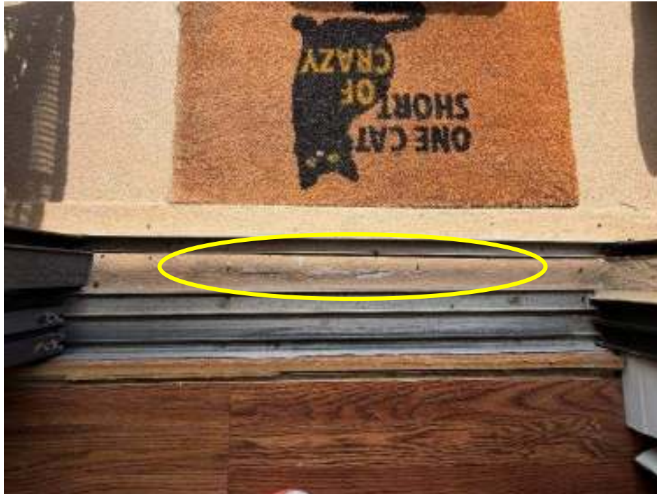
View of cracked door threshold, with likely spall located in slow below
