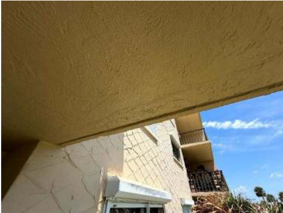
View of delaminated stucco
