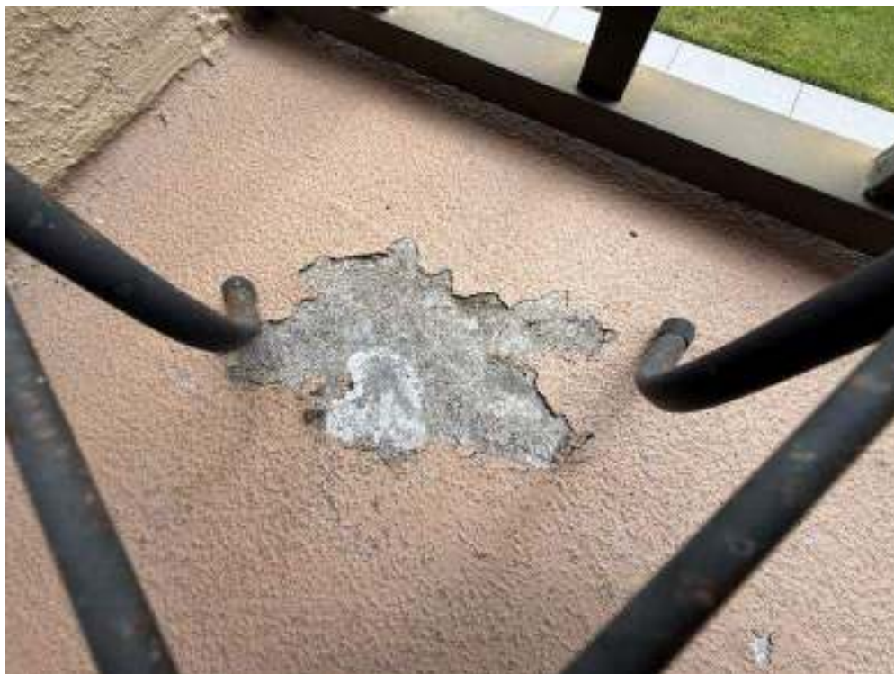
View of deteriorating coatings
