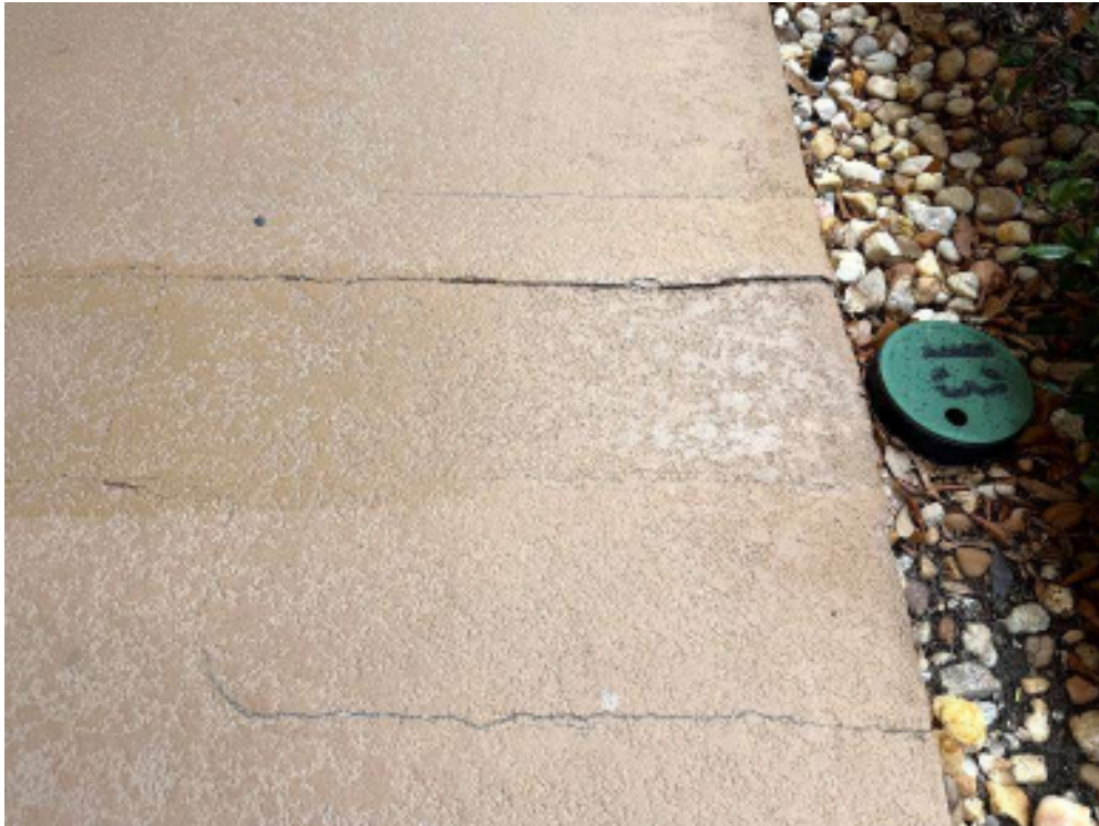
View of crack along ground floor walkway slab
