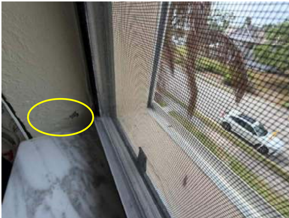
View of interior water damage at windowsill
