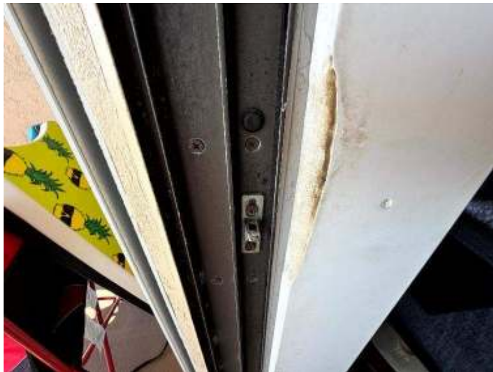
View of corroded sliding glass door fasteners
