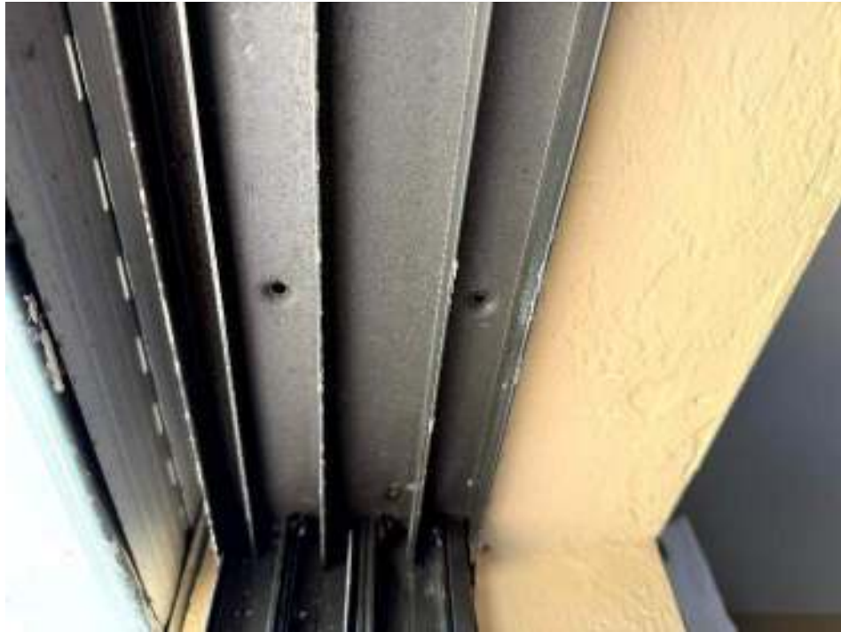
View of missing sliding glass door fasteners
