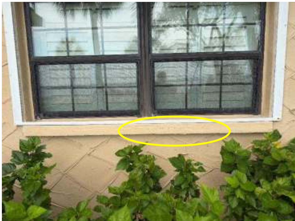
View of spalled windowsill due to reinforcing steel corrosion Note deteriorating window frame coatings
