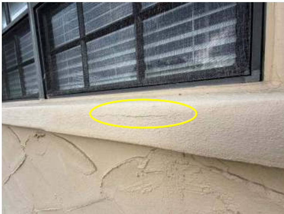
View of spalled windowsill due to reinforcing steel corrosion
