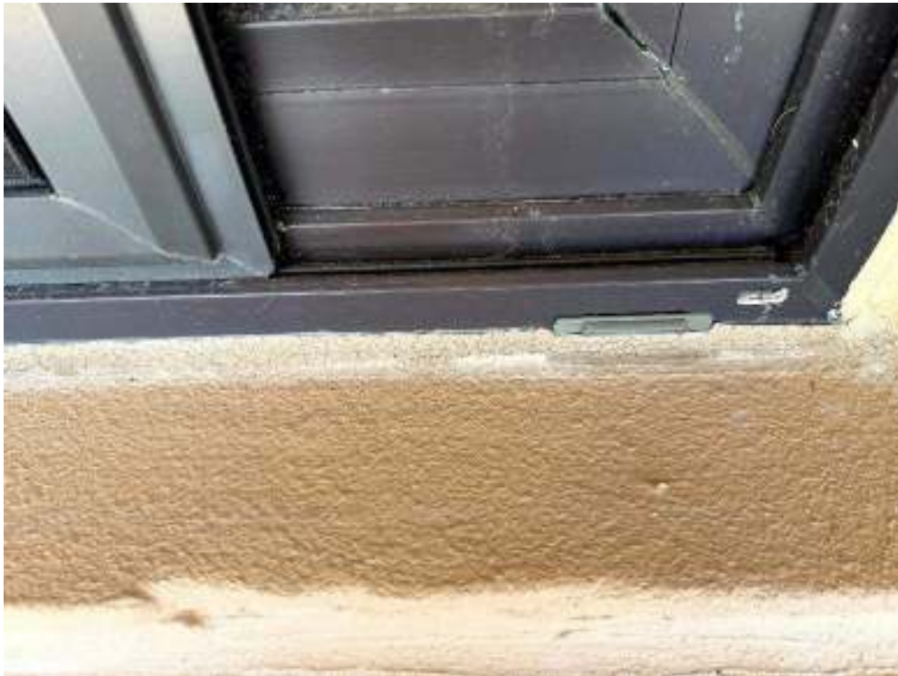
View of failing perimeter sealant at sliding glass door
