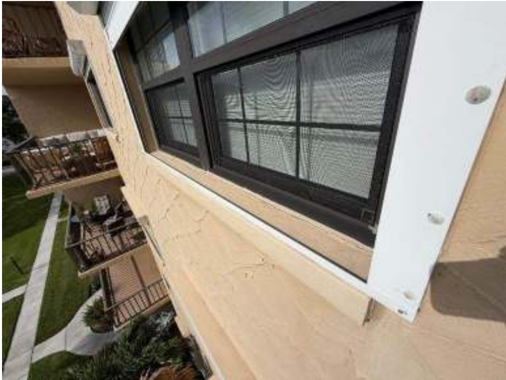
View of failing perimeter sealant
