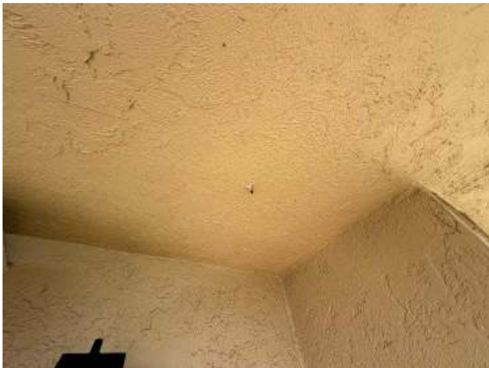
View of abandoned fastener in balcony ceiling
