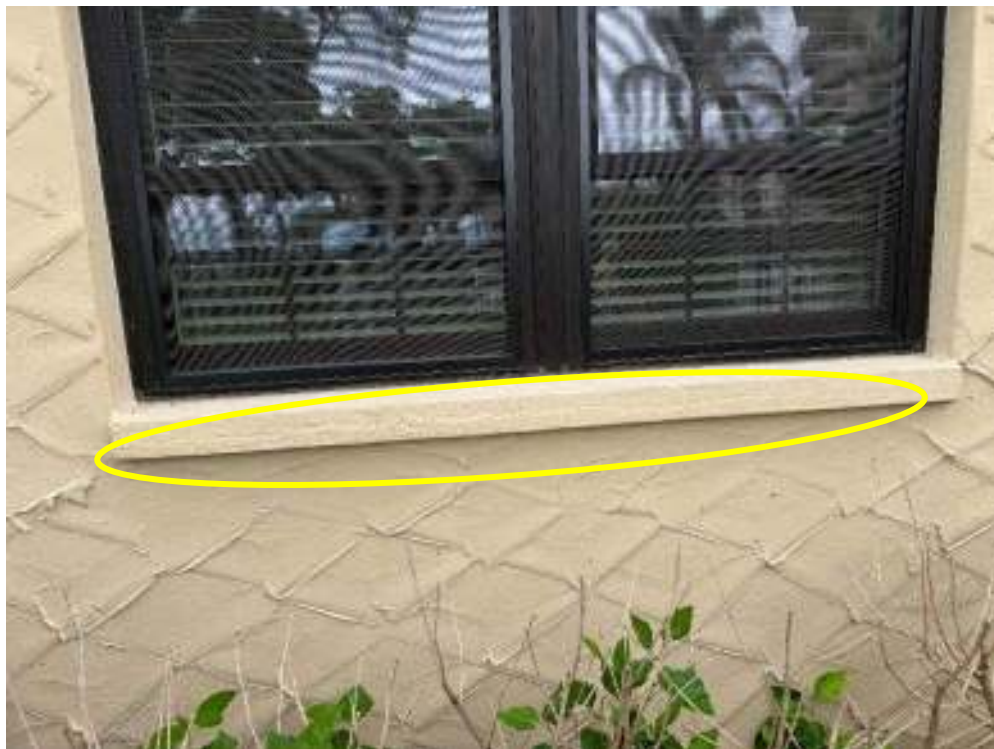
View of windowsill spall
