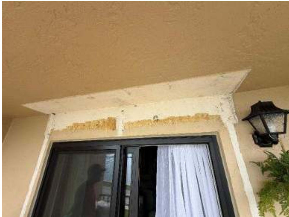
View of missing coatings at shutter removal area
