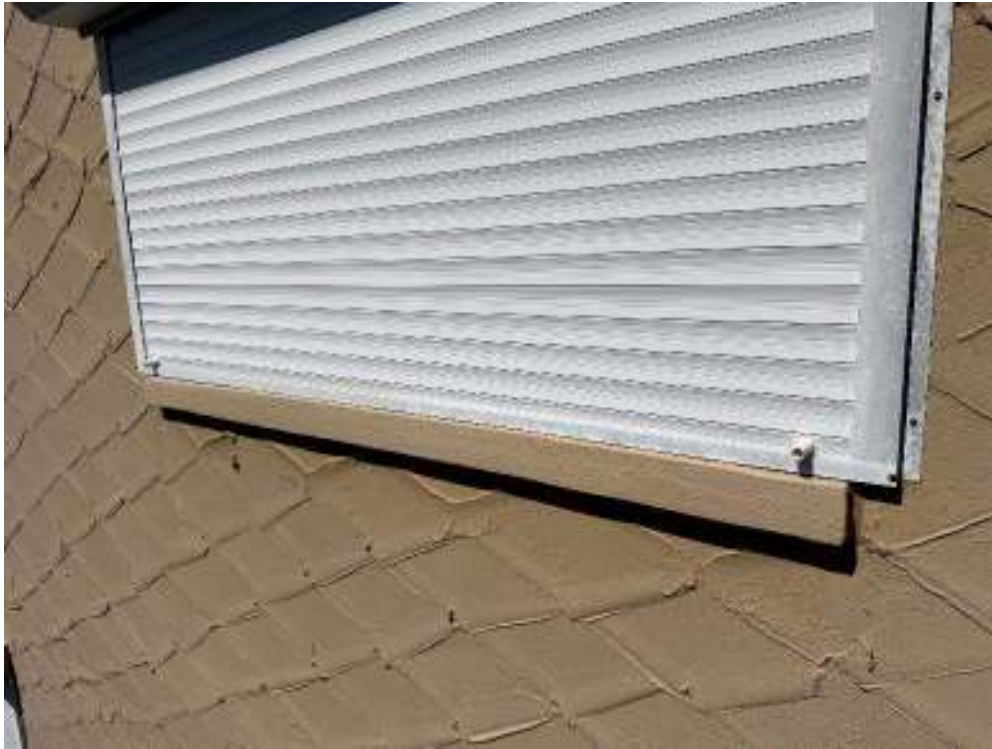
View of windowsill spall
