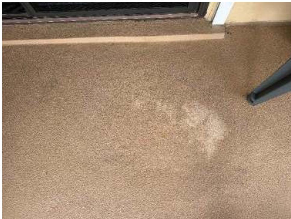
View of deteriorating coatings at previous patch
