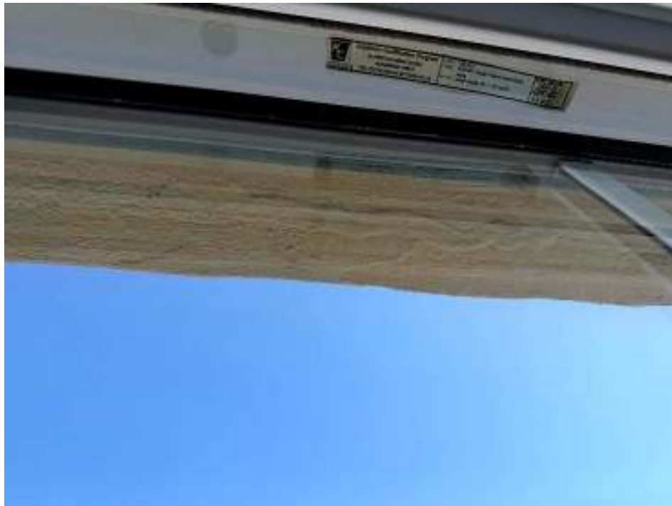
View of crack patch at window
