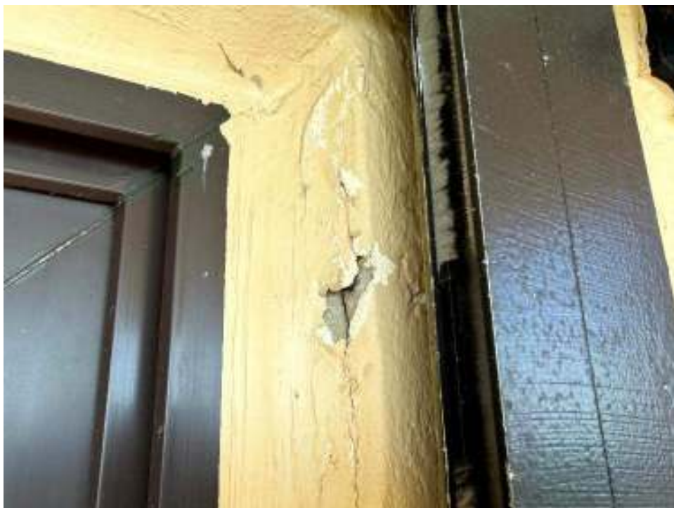
View of column spall due to reinforcing steel corrosion
