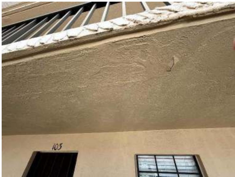
View of ceiling spall along ground floor walkway
