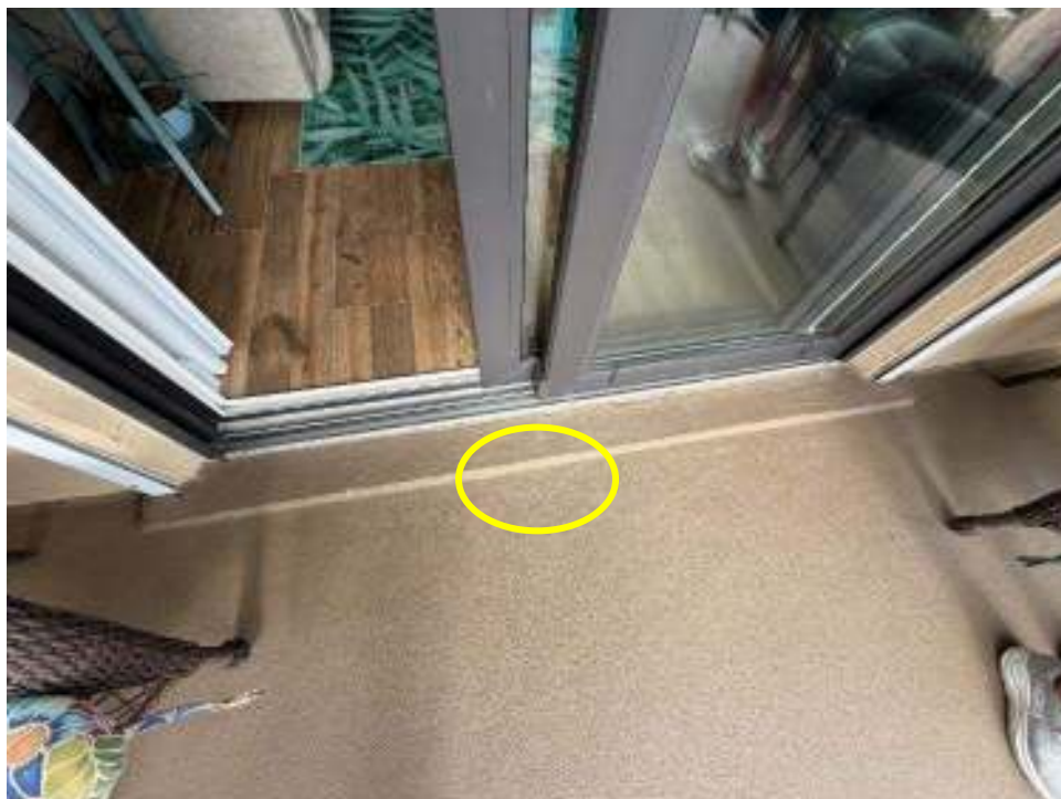
View of spall surface spall in front of door due to reinforcing steel corrosion
