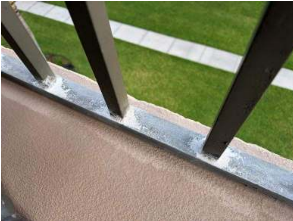
View of deteriorating railing coatings
