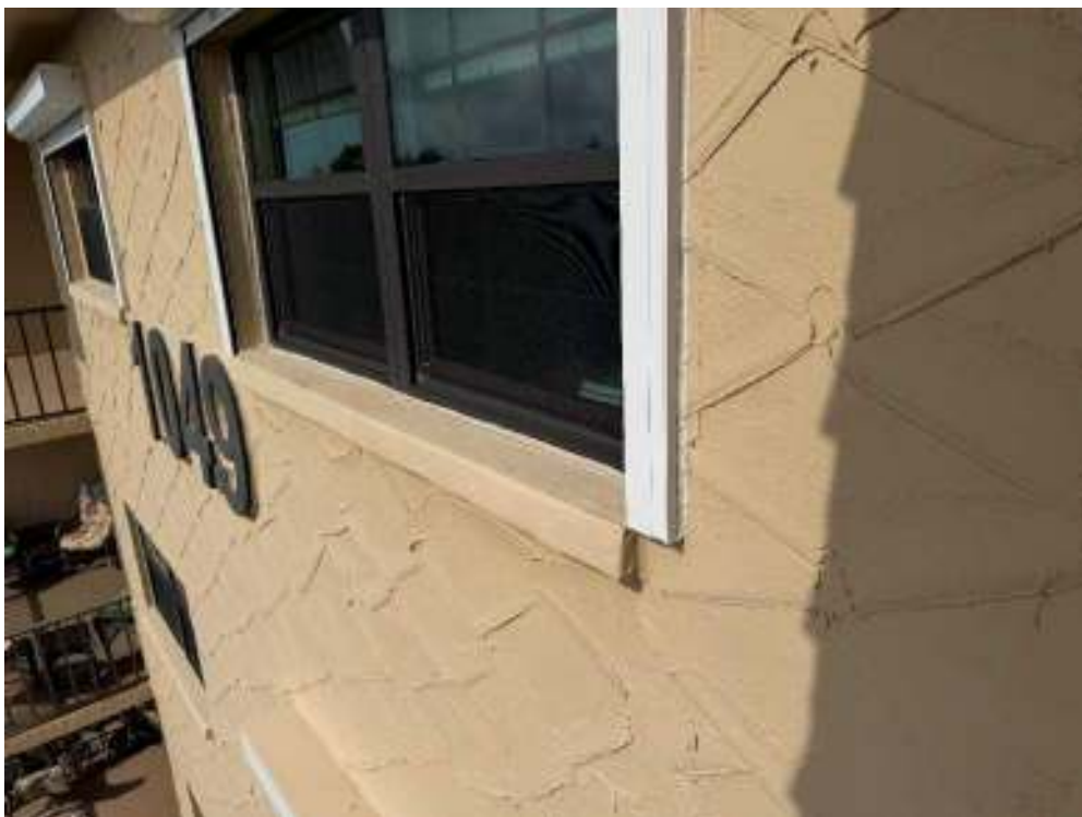
View of failing perimeter sealant
