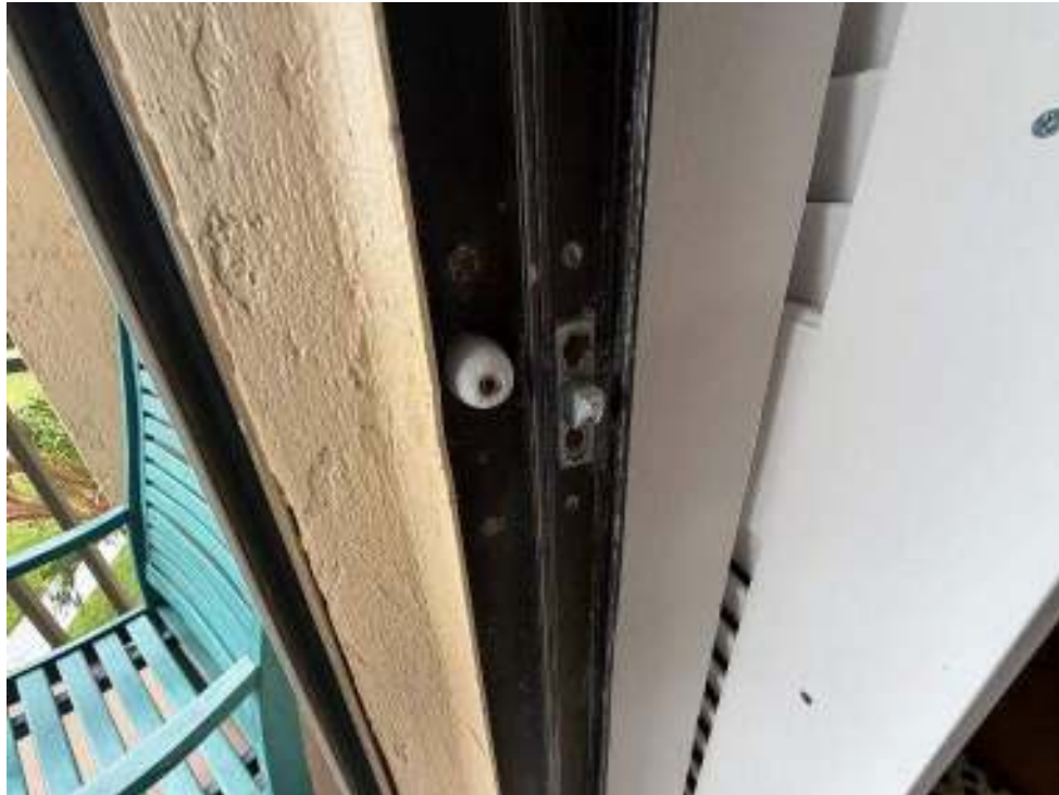
View of corroded sliding glass door fasteners
