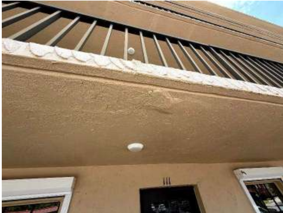
View of edge spall along ground floor ceiling walkway
