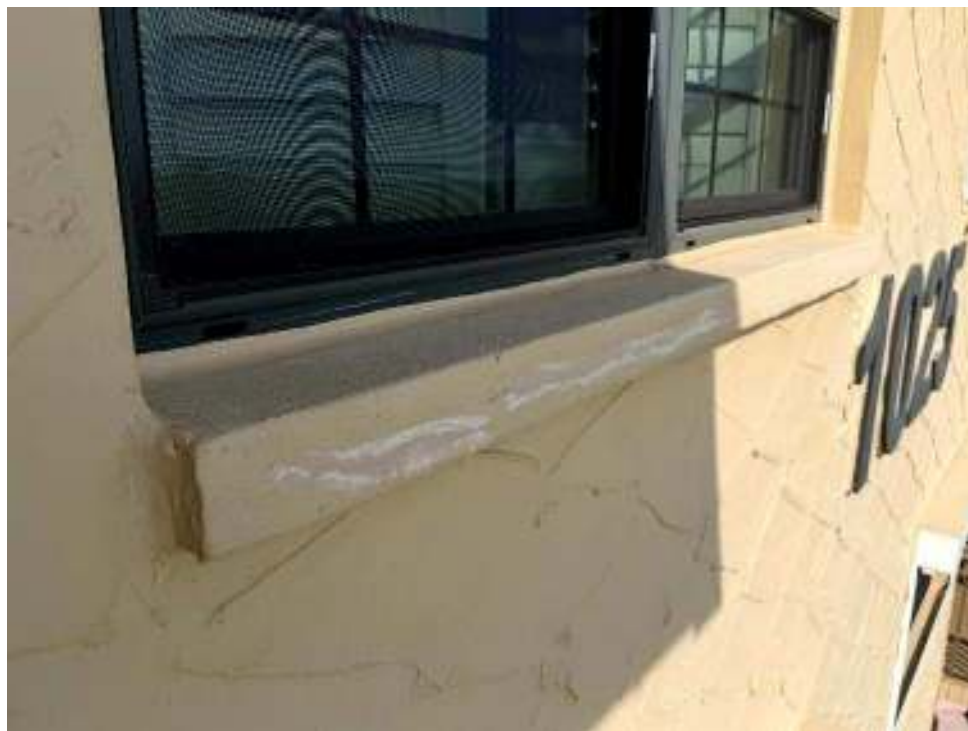
View of patched windowsill spall
