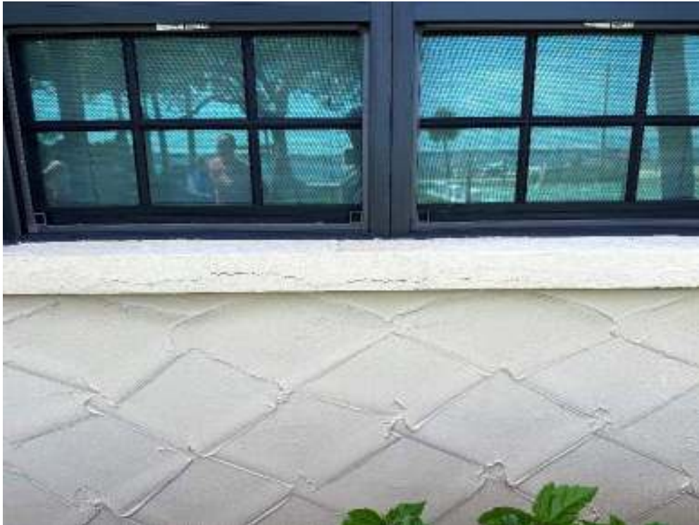
View of windowsill spall due to reinforcing steel corrosion
