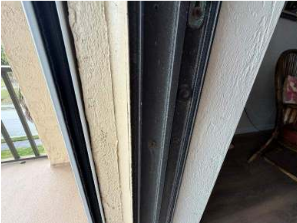
View of corroded and missing sliding glass door fasteners
