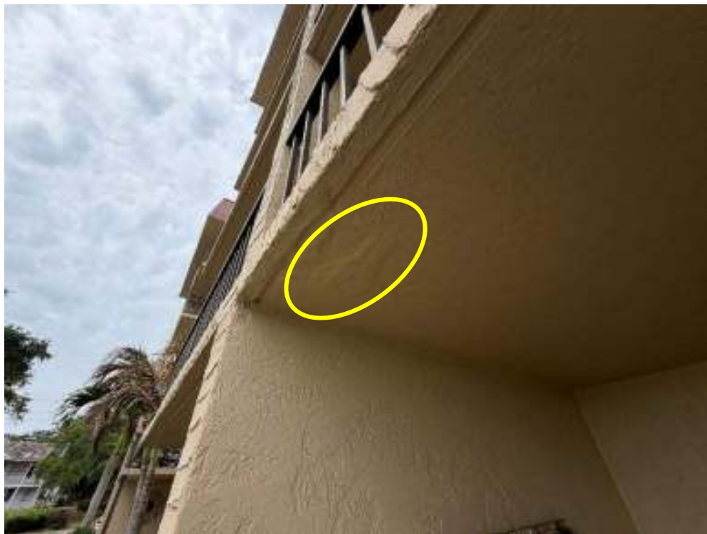
View of ceiling spall due to reinforcing steel corrosion
