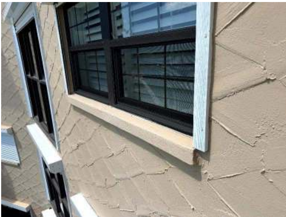
View of failing perimeter sealant at window
