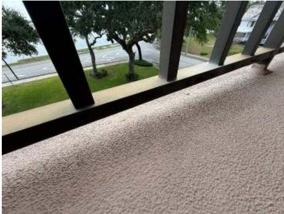
View of deteriorating railing coatings
