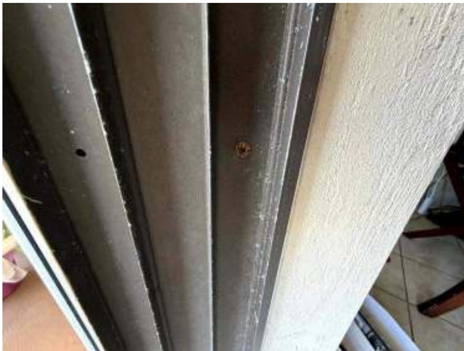
View of missing and corroded sliding glass doors fasteners
